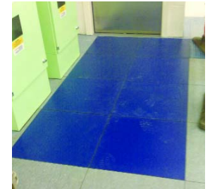
Dycem CleanZone installed directly onto access tiles inside the Royal Bank of Scotland mainframe room.
